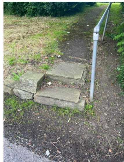
Inadequate access points
