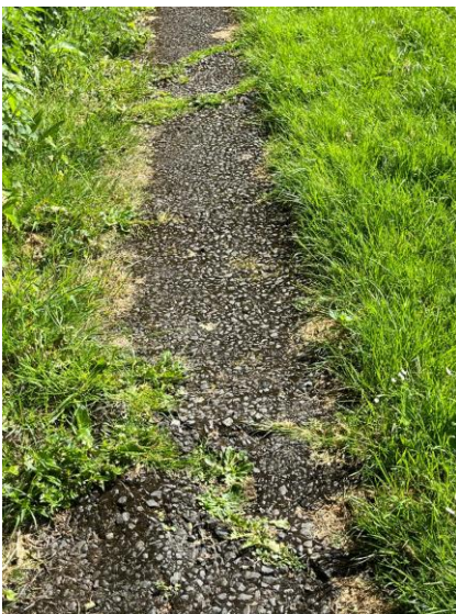
Poorly Maintained paths
